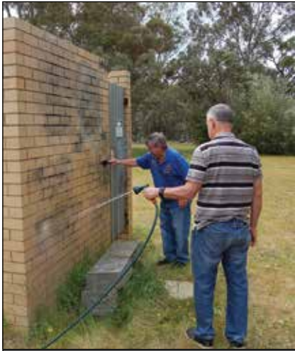
Graeme Whitehead scrubs while Bill Dunne hoses the wall down in the course of removing the graffiti.
