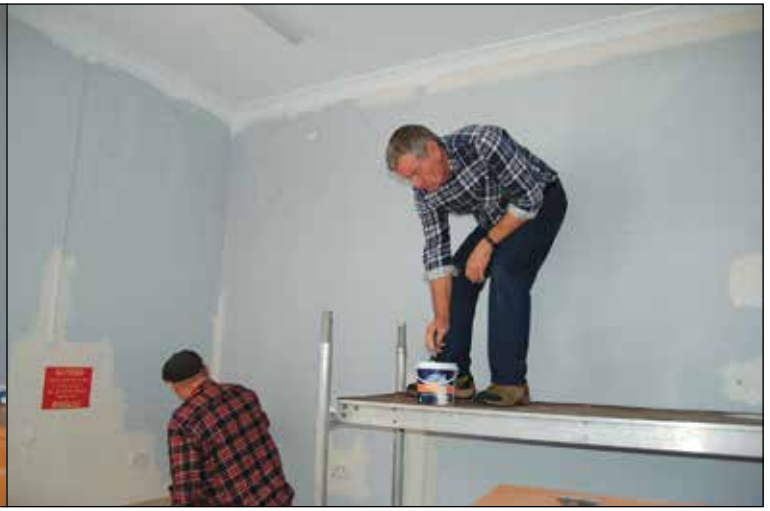
Chad Raven down low and Brian Eyre up high cutting in on the kitchen walls, September 29.
