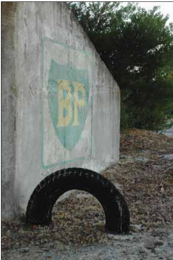
One of the footbridge abutments still carrying BP sponsorship. The marker tyre has lost its white paint over the years since 1968
