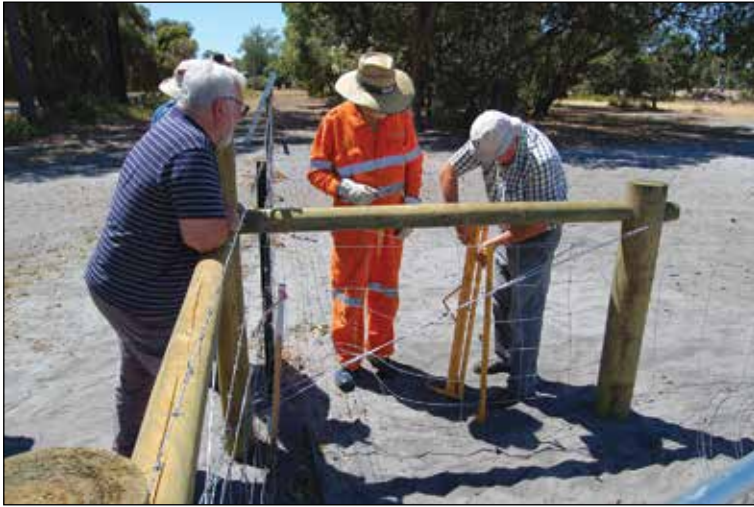
Glynn Allison, Kevin Dorn (obscured), Mark Jones and Barry Mackintosh stretching the fence around the building site.
