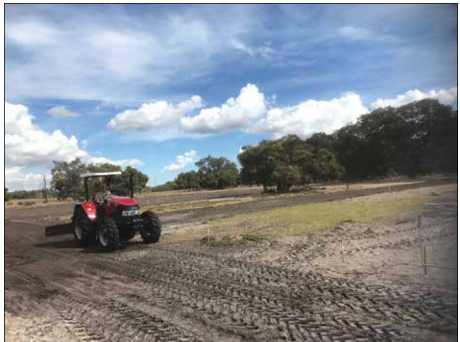
Barry Mackintosh finishing up with the pad area nicely cleaned up and the access drives prepared for Motivation Foundation.
