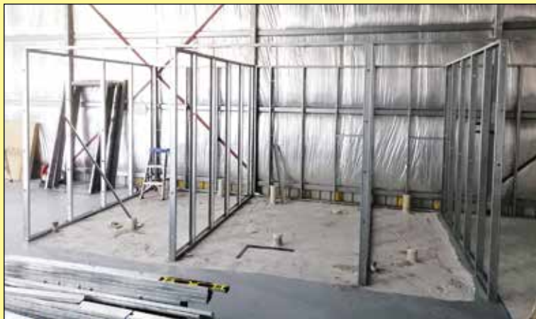
Above: The toilets framing after the first day of assembly on Dad's Army Tuesday, July 18.
