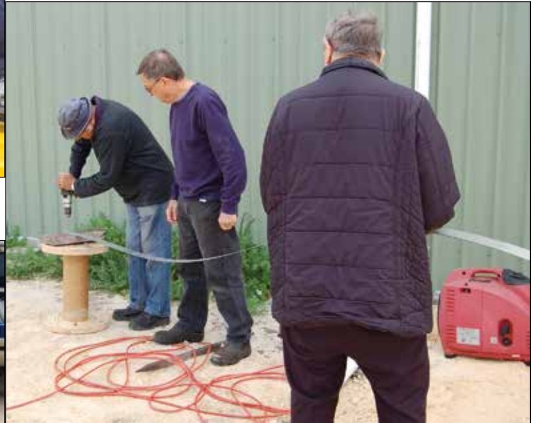
Ross Oxwell mans the drill, Nick Danielle looks on and Wally Phoebe holds the metal strip, preparing parts.
