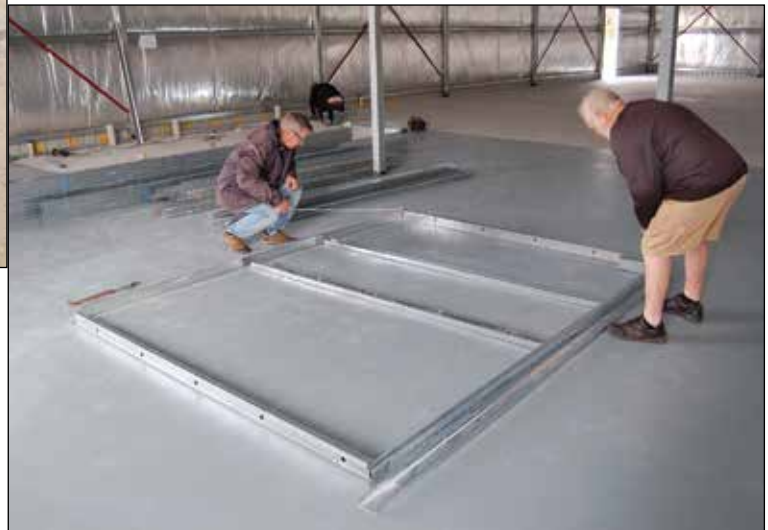
Brian Eyre and Kevin Dorn measure up the first of the frames while Graeme Whitehead works in the background
