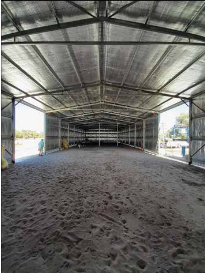
The interior of the clubroom building before the concrete was poured. It looks vast, but it won't take long to fill it up, with the help of VSCC volunteers.
